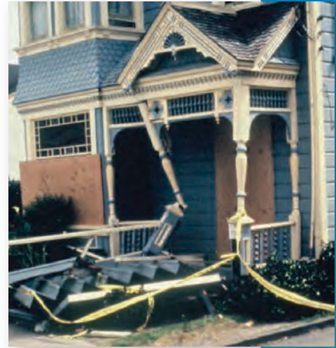
This older home collapsed after earthquake shaking damaged its crawl space (cripple) walls.
